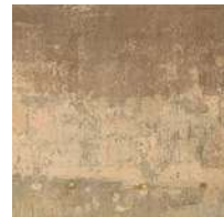
Weathered Concrete Walls Surfaces
