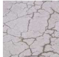
Weathered Concrete flooring
