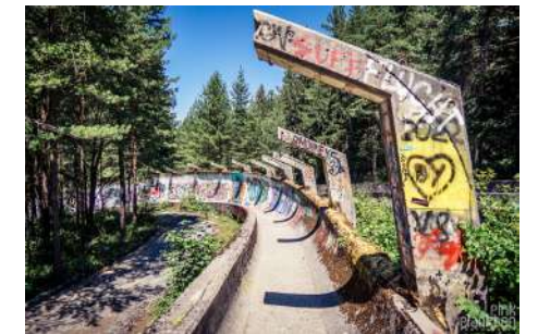
(046) Physical Concrete Support for Sarajevo Bobsled Run, Built in 1984, Photographed in 2024 Gorazd Bucar, Concrete, (~ 12' x 8' x 2.5")
