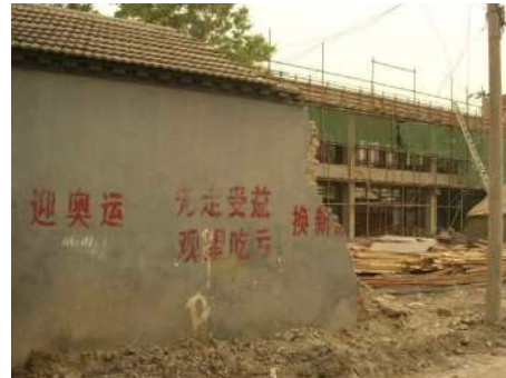
(067) Hutong Marked for Demolition (text reads "Welcome the Olympics, Leave early receive early benefits, Wait around lose out"), 2008 Unknown Maker, Spraypaint, (120" x 36")
